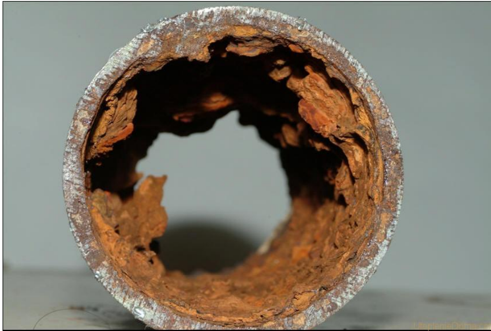
Fig.7. Rust in the pipe.
